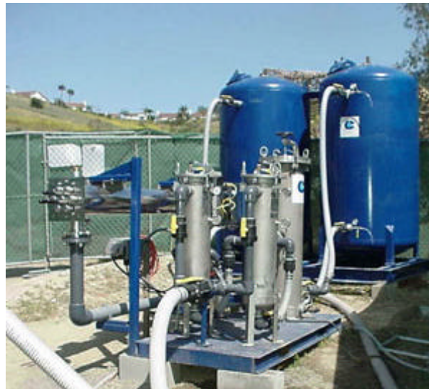
Figure E1-37 Clear Creek UV System
