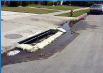
Sandbags blocking an inlet and causing a safety hazard
