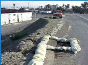
Sandbags blocking inlet and causing a safety hazard
