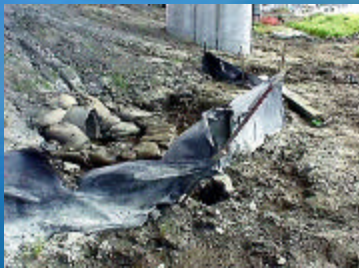
Incorrect use of silt fence
