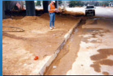
Lack of sediment control
