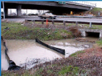
Silt fence installed incorrectly in a concentrated flow area
