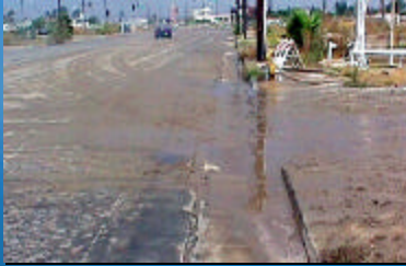
Lack of stabilized entrance / exit
