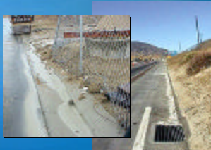
Uncontrolled concrete washouts
