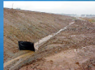
Silt fence installed incorrectly in a un-stabilized concentrated flow area
