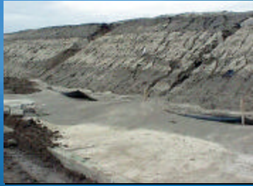
Lack of soil stabilization has led to failure of silt fence
