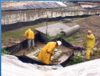
Maintenance of BMPs is a critical requirement for an effective water pollution control program
