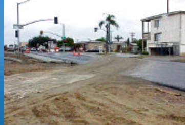
Lack of stabilized entrance / exit
