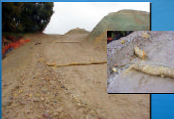
Incorrect installation of fiber rolls; too far apart, not trenched in
